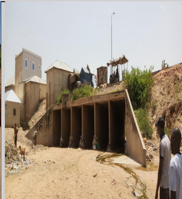
Figure 2.6: Existing Culvert along the gully stretch in Downstream of FCE (Tech) gully site at Arawa 'B'
